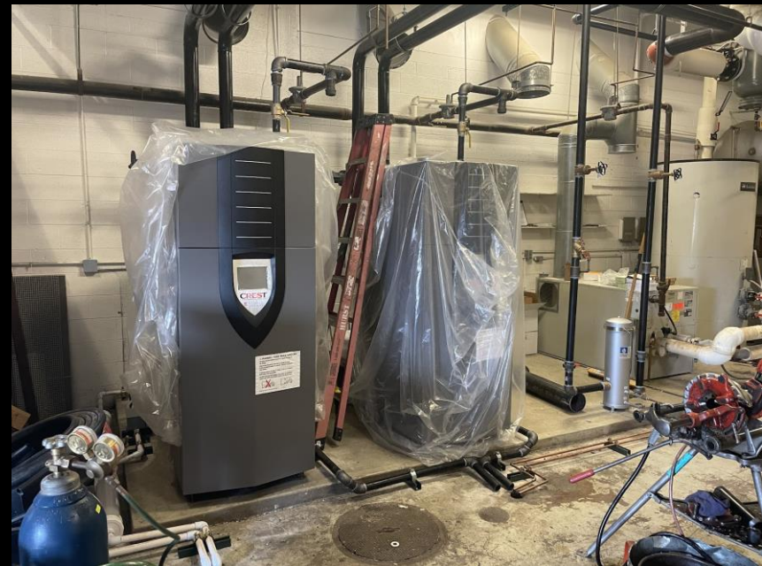
MIDDLE SCHOOL BOILERS
