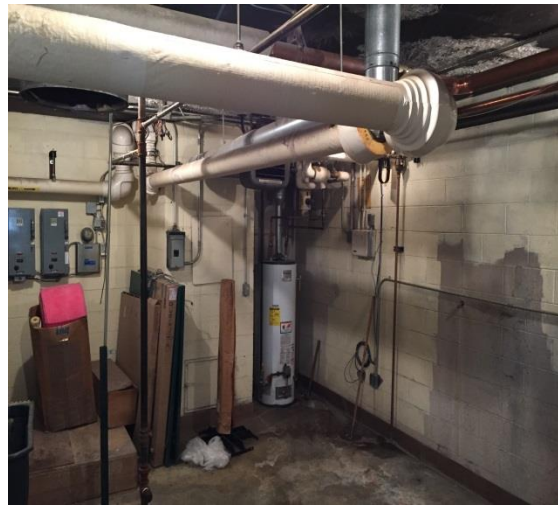
Explorer Elementary Boiler Replacement $34,300
